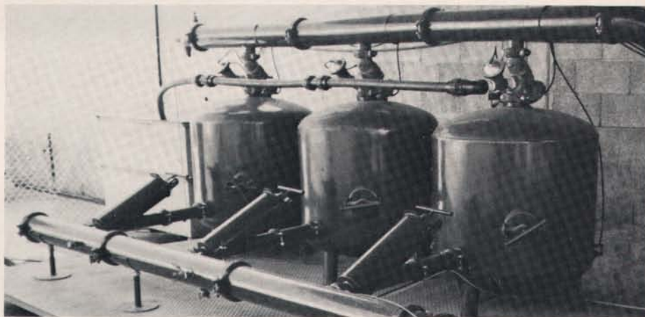
Three-barrel media filter capable of 800 gallons per minute. Photo courtesy: Efco.
