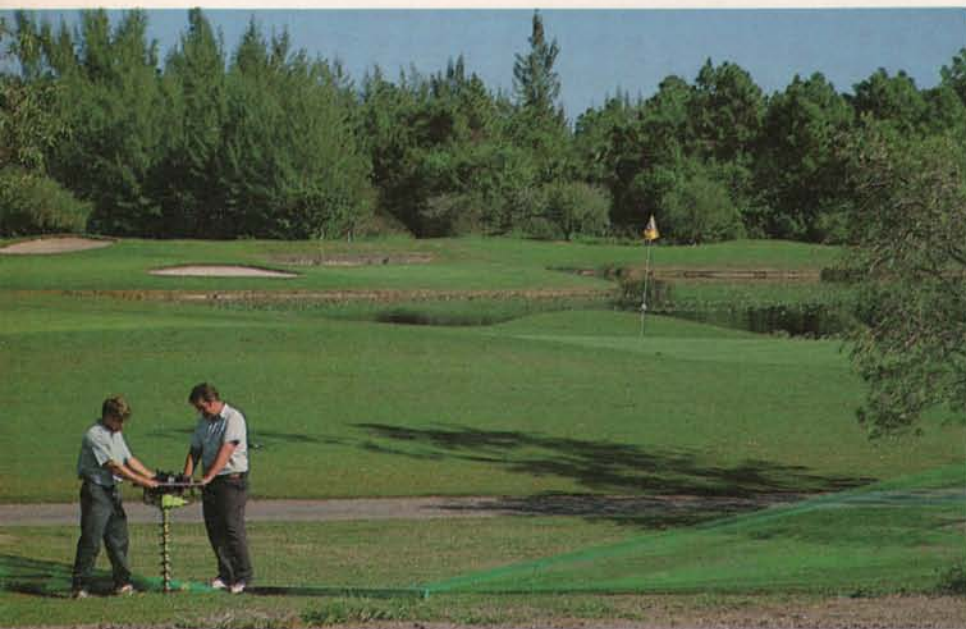
The PGA National crew drills holes for posts to hold erosion fence around the perimeter of the Champion course.
