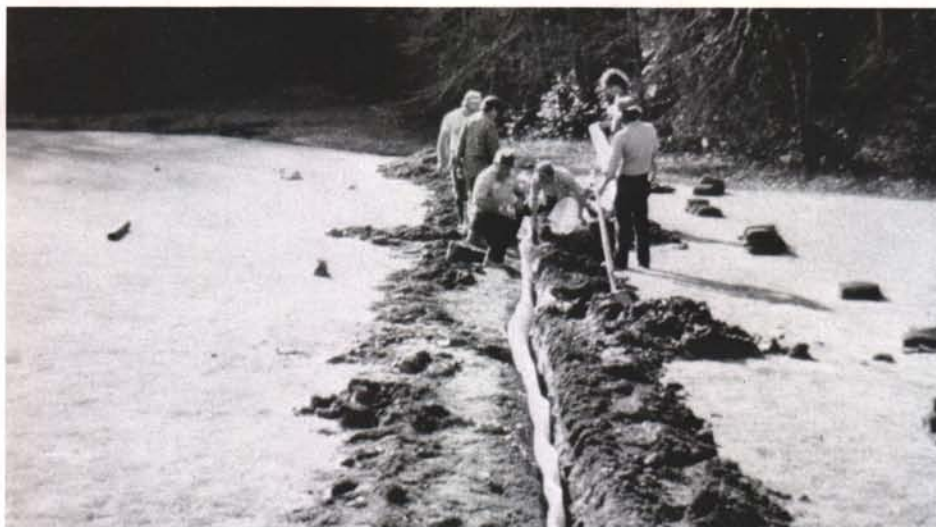
Enkadrain H was installed on top of drain tile in trenches across the seventeenth fairway.
