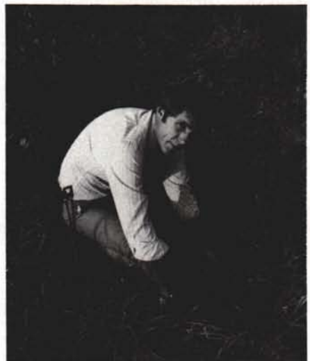
Clint Granath lifts one of the PVC mainlines hidden beneath the turf.
