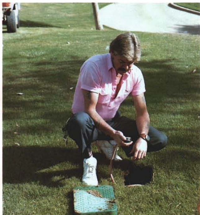
Richards Jenkins, irrigation supervisor at Gainey Ranch, checks the valve output pressure to the heads.
