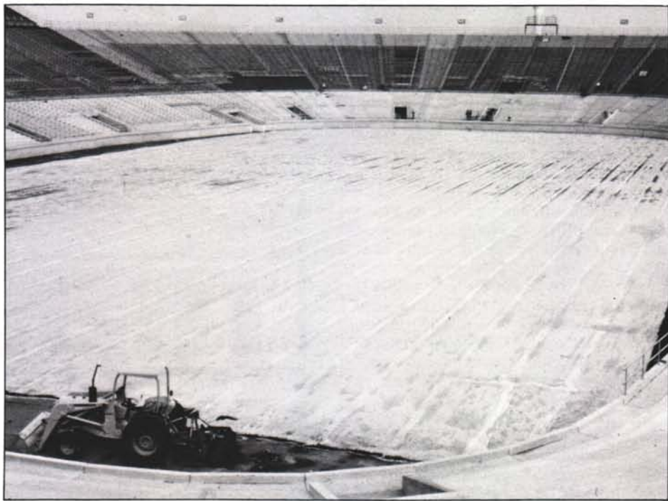
Fumigation of soil prior to establishment can greatly reduce future weed problems.
