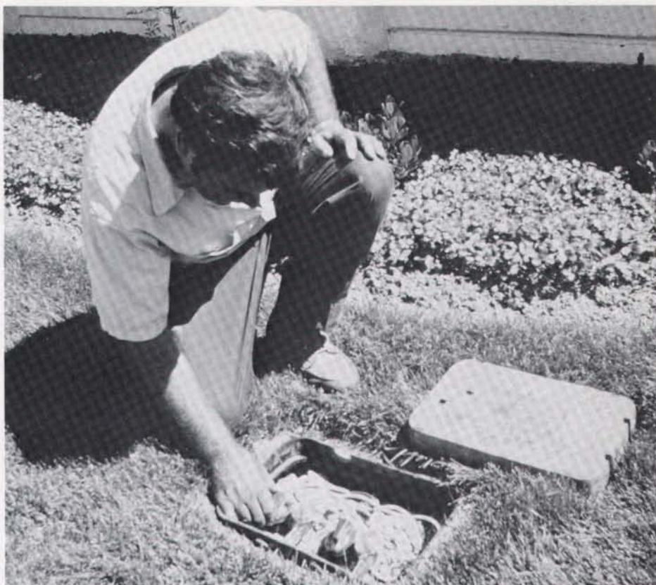
Irrigation manager sets the switches on the moisture sensing devices for the desired moisture levels.
