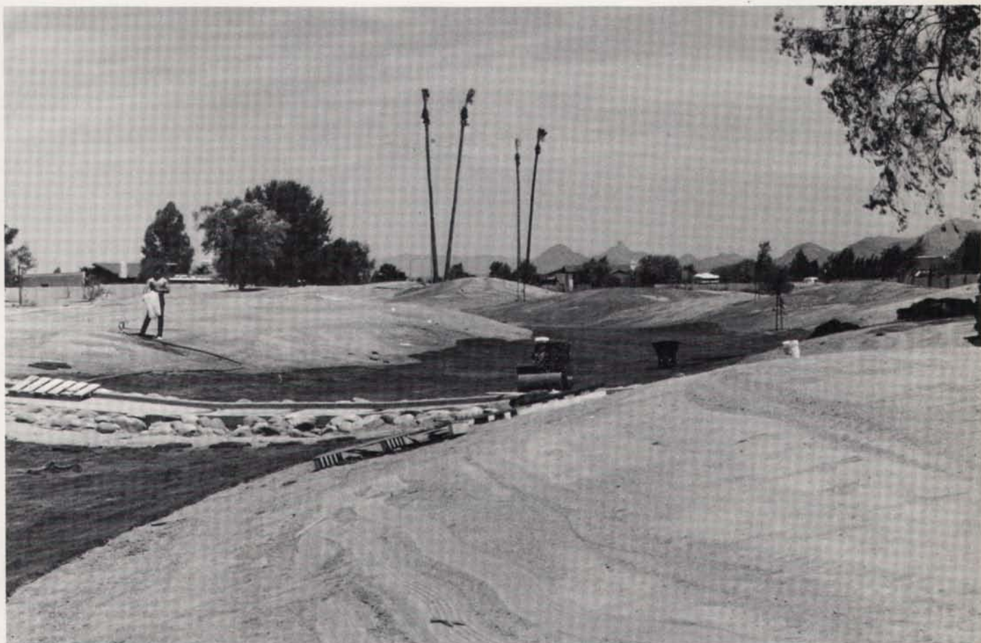
More than 45,000 sq. ft. of bermudagrass sod was installed in drainage channels in one 10-hour day.
