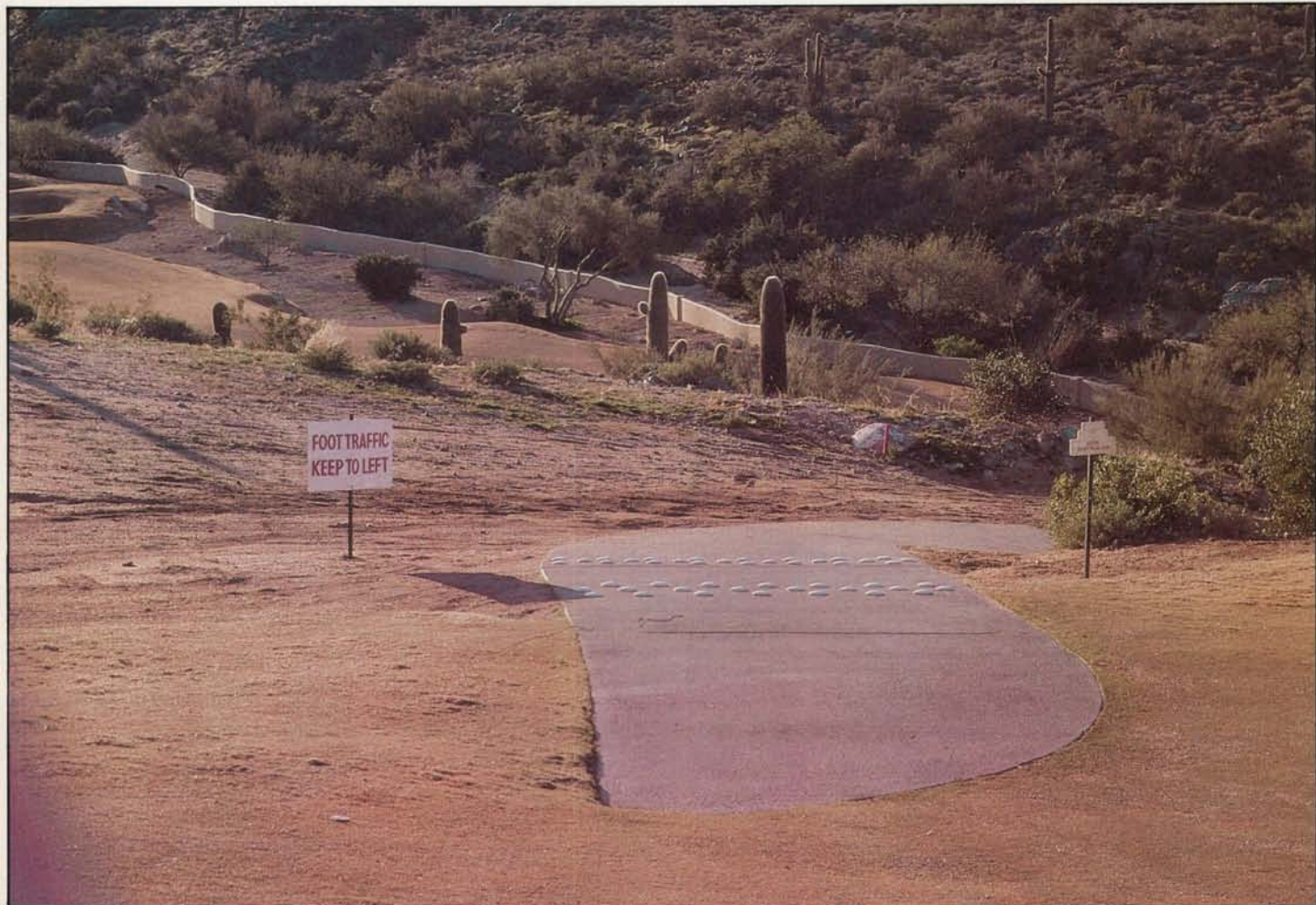
Quarter-circles at the end of cart paths disperse golf cars exiting from the path and help reduce concentration of wear.
