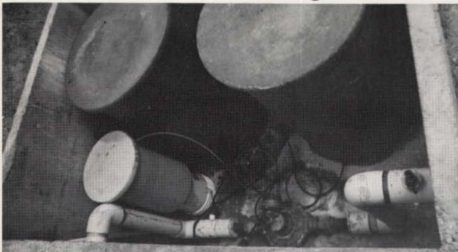
Tanks for liquid fertilizer and injectors in underground vault.
